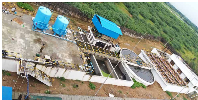
Figure 2.11: An effluent treatment plant in Tamil Nadu. (Water Care Equipments & Services, 2024)
